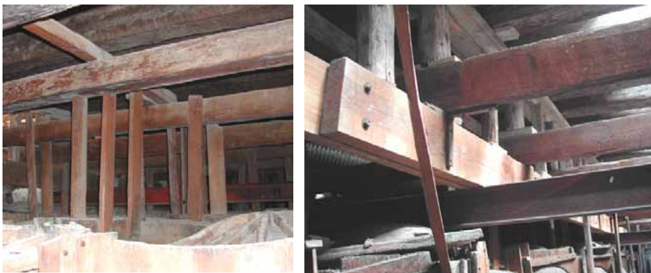
Fig. 5 – The articulated system that support the muqarnas ceiling, constituted by hemi-squared wooden beam with wooden tie rods and reinforcing wooden beams ( rompitratte ), NP16 steel beams.
