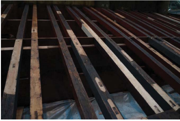
Fig.4 Different kinds of repairs of rafters made by splicing damaged timber with new wood, Rin'oji Temple, 2015. The date of the repair is burnt into the new.
