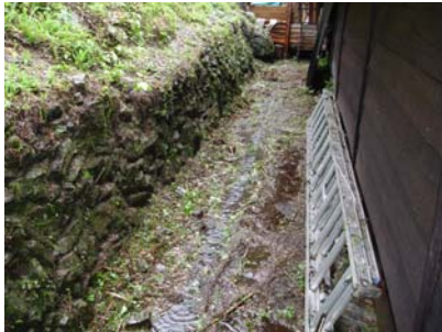
Figure 9. North side depression
