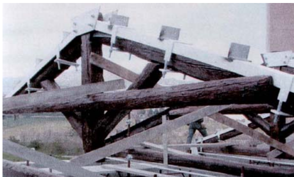
Figure 18. The angle braces on the channel irons used to haed secondary beam
