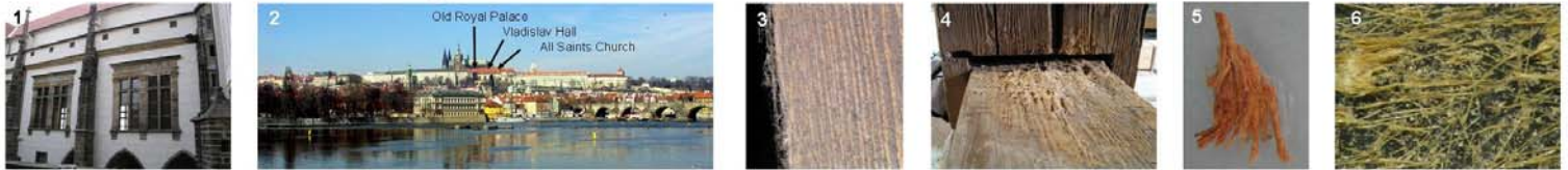
Figure 1 – View on the Vladislav Hall building. Figure 2 – View on Prague Castle. Figure 3 – fine fibers on wood surface has appeared again after conservation treatment. Figure 4 – The most damaged timber above the Vladislav Hall. Figure 5 – Detail of the corroded wood from the figure 4. Figure 6 – Fiber sample taken by tape from the wood surface.
