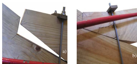
Figure 21. Joints with tension ties: a) contact loss on the front surface (closing skew angle); b) failure due to stresses perpendicular to grain (opening skew angle)
