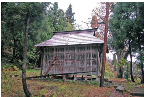
Figure 1-1. Juni-jinja shrine just after the earthquake in 2004
