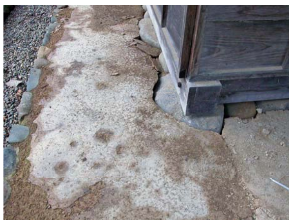
Figure 2-2. Subsidence of foundations in Hasegawa-family house by the earthquake in 2004
