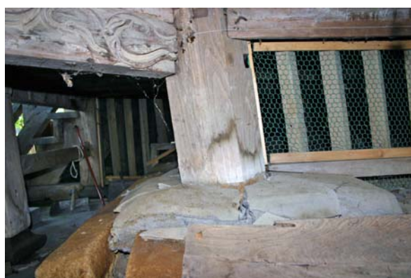
Figure 3-2. Inclination of the post in Tata-jinja shrine by the earthquake in 2007
