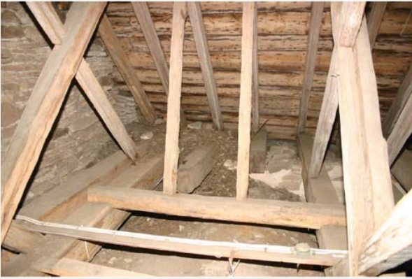
Figure 6 Marka church. a) and b) Rot damages. c) Tie beams have been cut off and struts removed where vaults are built in. Extra parts have been added to compensate for lost ones. Photos: Carl Thelin.
