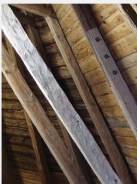
Figure 4 a) Repair measures: a new part (in the foreground) and a spliced rafter. b) New wall plates and new rafter ends. The picture was taken when the whole structure was lifted by jacks in order for one of the beams to be replaced.
