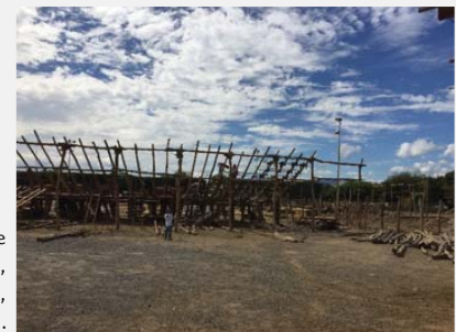
Picture 8. The structure in process, Ivonne Calvillo, Villa de Álvarez, Colima, february 2016.
